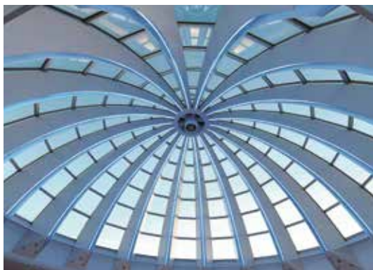
The area beneath the dome of the Further Education Centre is generous and spacious
